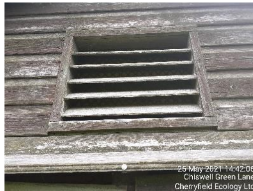
Figure 21: Example of louvre window which has been sealed internally.
