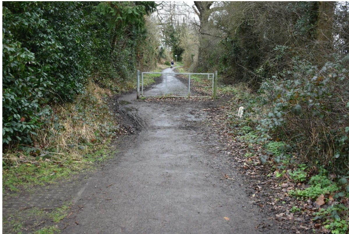
Nightingale Lane near A414 showing the state of surface and barriers across the route.
