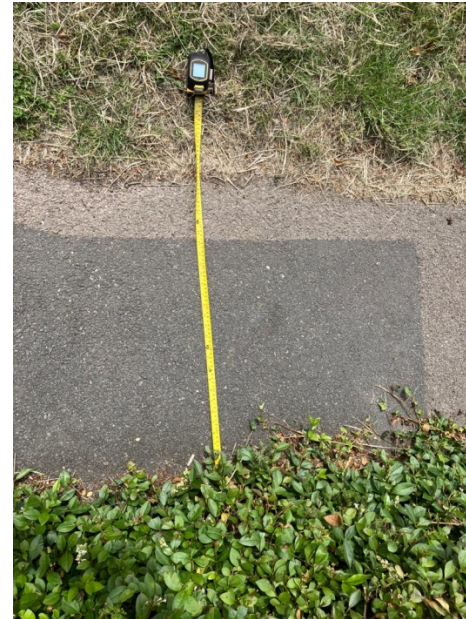
Old and crumbling surface
