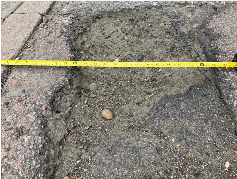
60 cm width from brick wall to kerbside (see also White HGV below)
