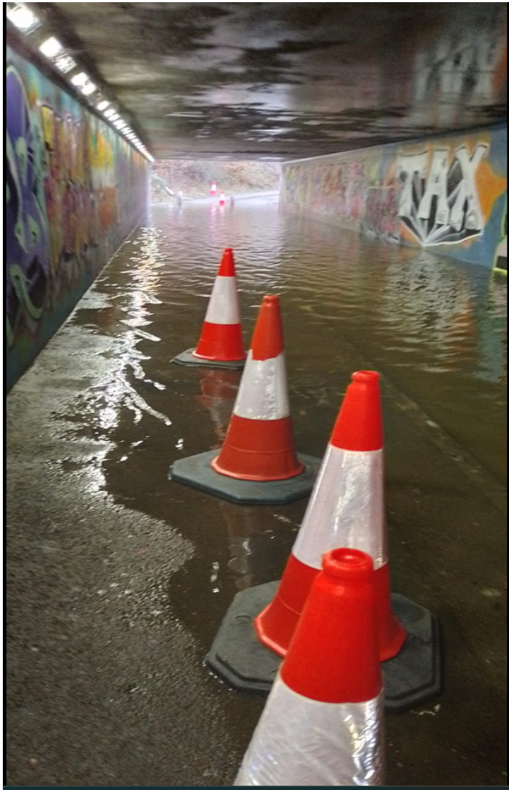
A1(M) subway Bullen Green Lane to South Hatfield flooding January 2023
