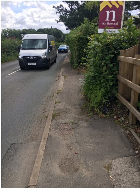
Poor pavement surface and extreme narrowing of width
